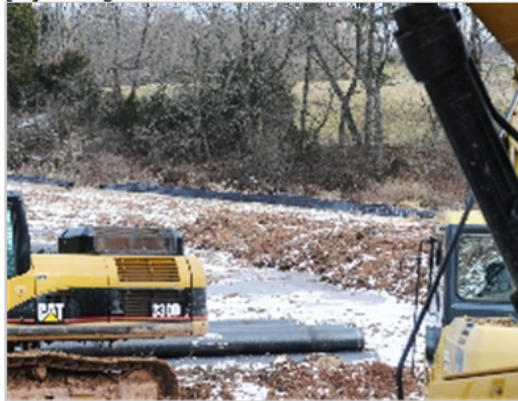
Reading Eagle: Susan L. Angstadt Work on a 3-mile extension of the Amity Township sewer system is visible from Route 422 near Baumstown. Township officials expect the project to be tested and certified by early May.
