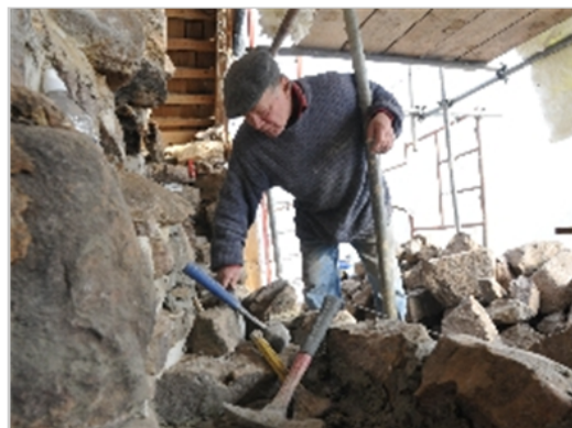
Reading Eagle: Bill Uhrich + MORE Joe Forrest of Port Royal, Juniata County, works on restoring the stonework in the Bridge Keeper's House at Morlatton Village, near Douglassville.
